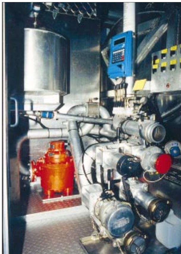
Fig. 2 Control room and pipe fittings
